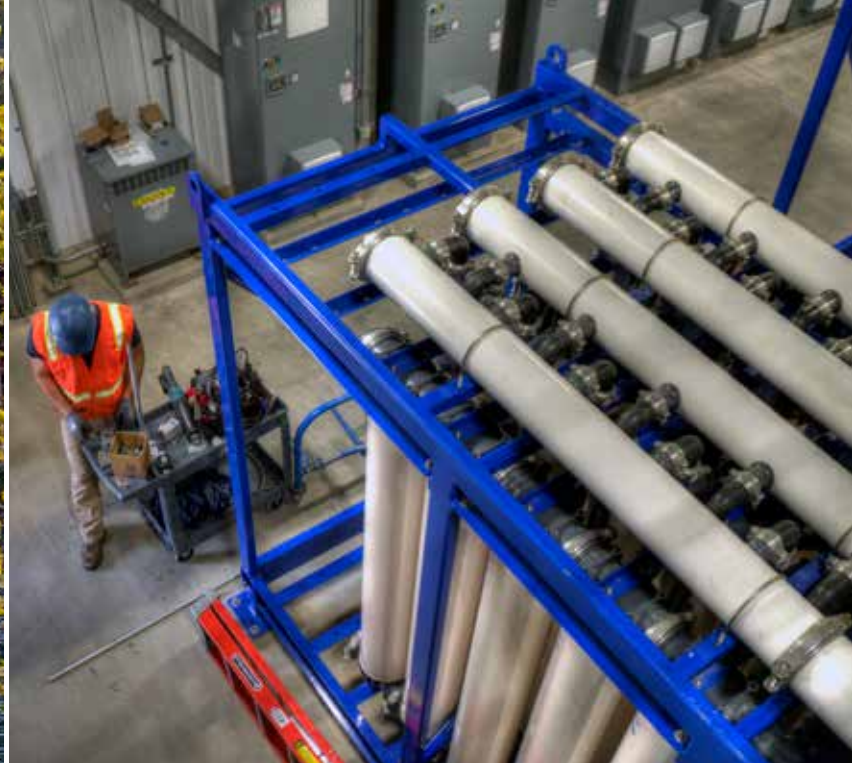
Ultrafiltration modules, like the one shown above, remove parasites, bacteria, and viruses from the water.
